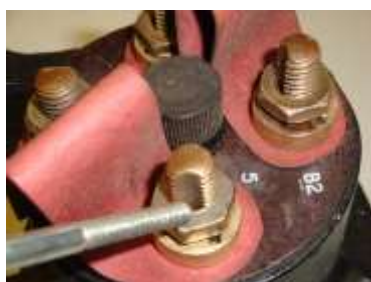
All terminals are marked but not always as clearly as this
