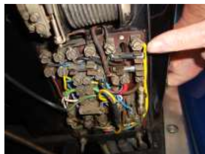
Main fuse is horizontal
