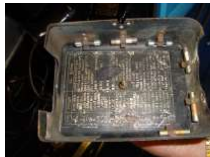
Inside the fuse box lid. Note spare fuses
