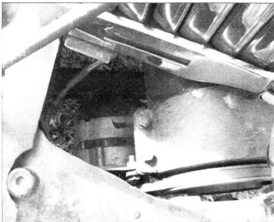
Above: A pulley fitted on the end of the dynamotor driving an alternator mounted underneath it.
