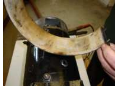
Check paper insulation is intact
